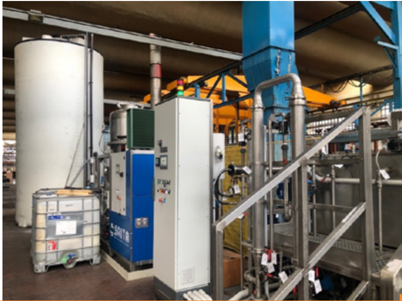
Figure 1 - ultrafiltration and distillation plant in operation in CleanAir Europe Srl
